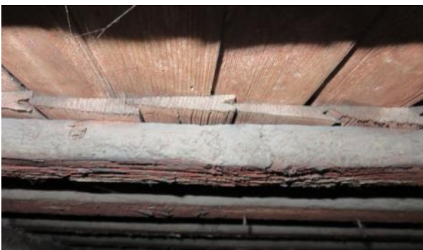
Figure 8: Detail of the tongue and groove wooden shingles, which have survived over a large area beneath a recent cement-asbestos covering. Haidgasse 6, 1020 Vienna, 2016 (BDA Liebich)
